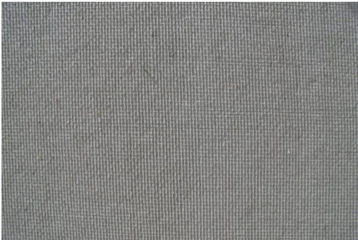
Figure 1: Close up view of the texture of a fabric formed concrete wall.
